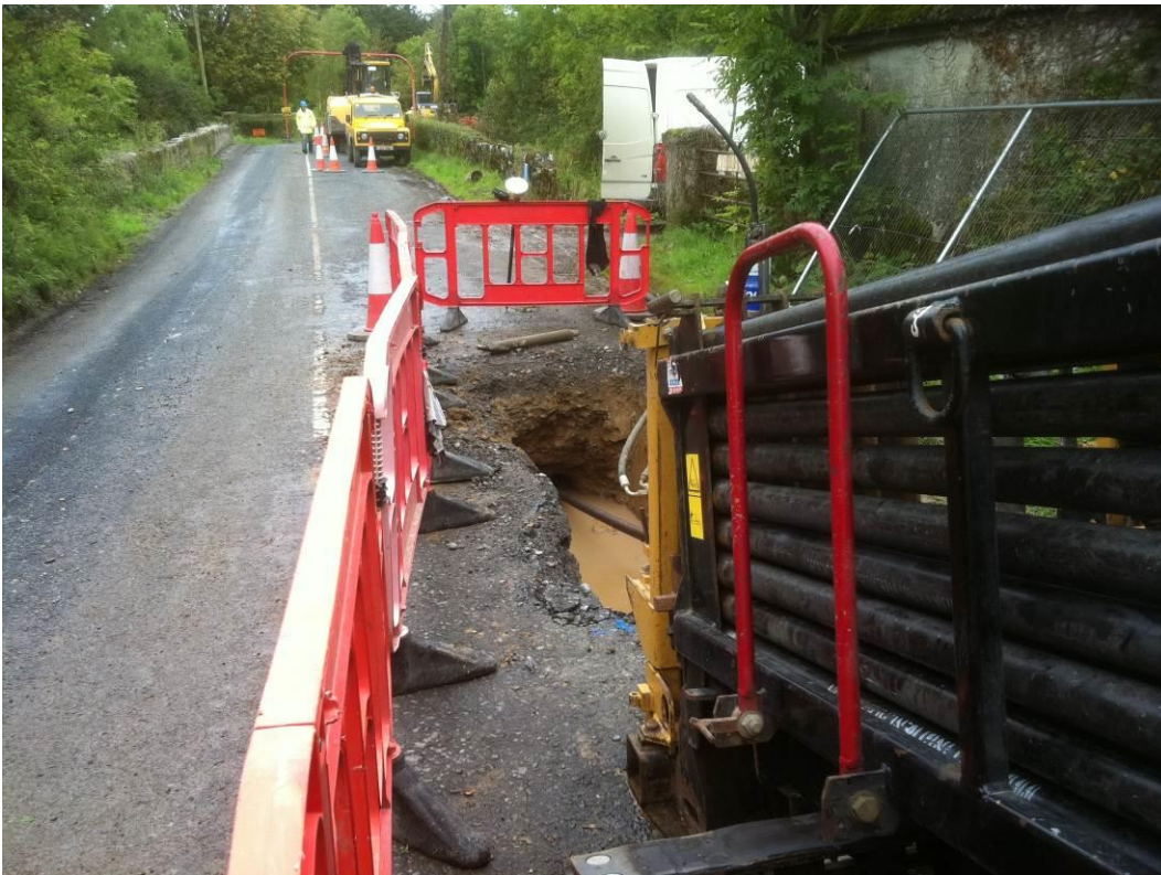
Figure 7: Standard HDD site on local road where HDD was used to go underneath a bridge (bridge parapet walls visible)
