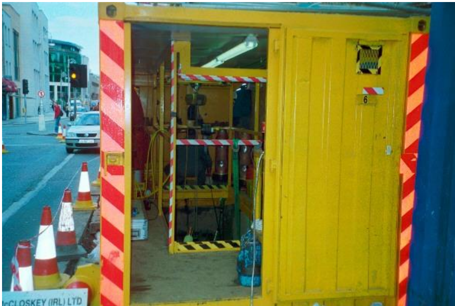
Figure 15 : HV cable jointing container
